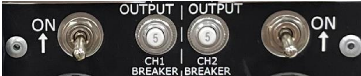
Figure 4: Channel controller power switches and breakers.
